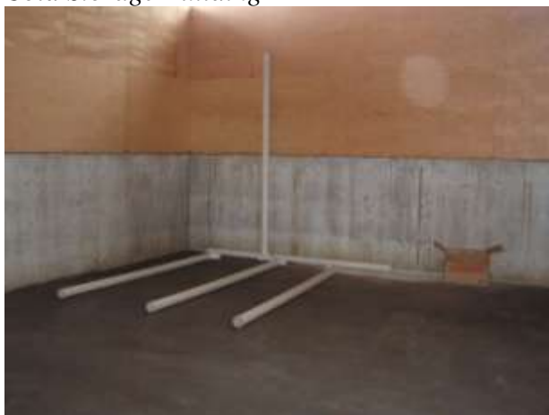
Gunter Bros. Meat Co. Compost Building With Aerated Floor
