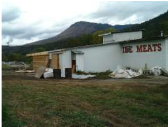
Riverside Natural Meats Refrigerated Waste Storage Room
