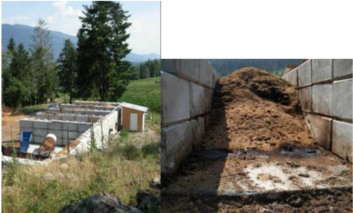
Rainer Farm Bin style Compost Containment With Aerated Floor. Computerized Blower System in Shed.
