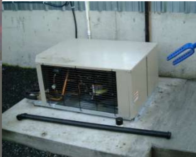
Cooling Condenser Unit for Storage Room
